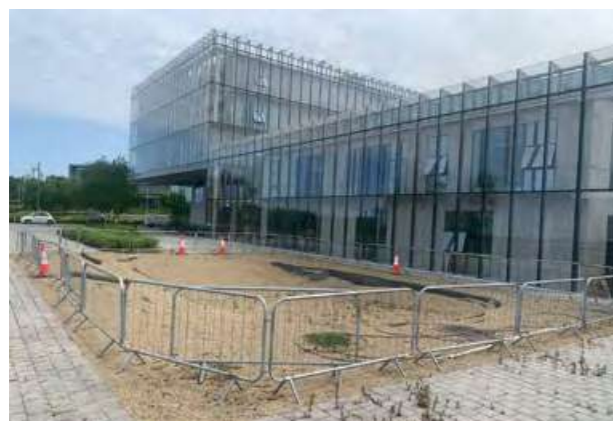
Figure 22: Collapsed Attenuation Tank - Wexford County Council
