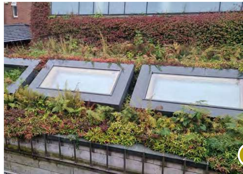
Figure 18: Green Roof - Engineers Ireland, Clyde Road, Dublin
