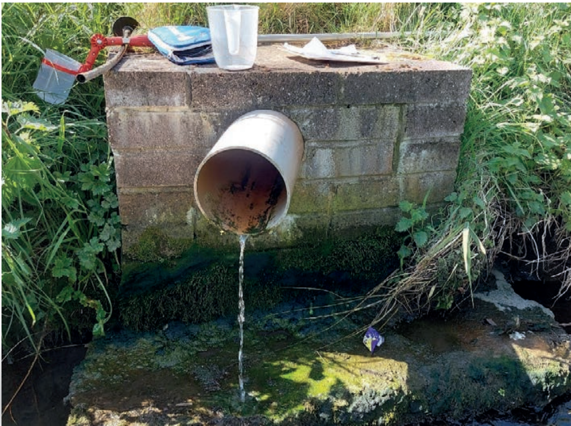
Sampled pipe inflow discharging to the Santry River.
