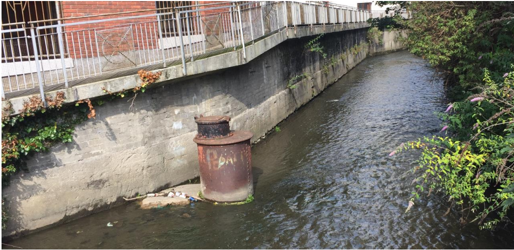
Figure 25: Example of sewer infrastructure acting as a hydromorphological pressure
