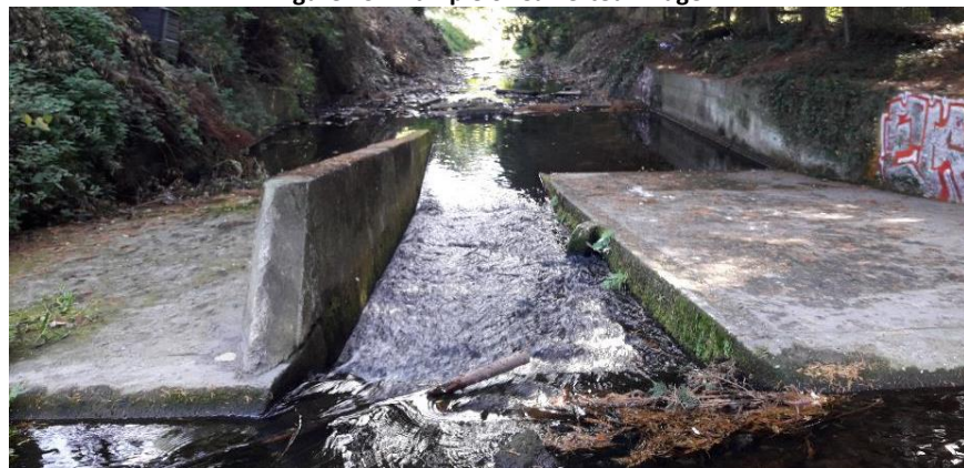
Figure 24: Example of old structure (perhaps on old mill structure) not removed from river
