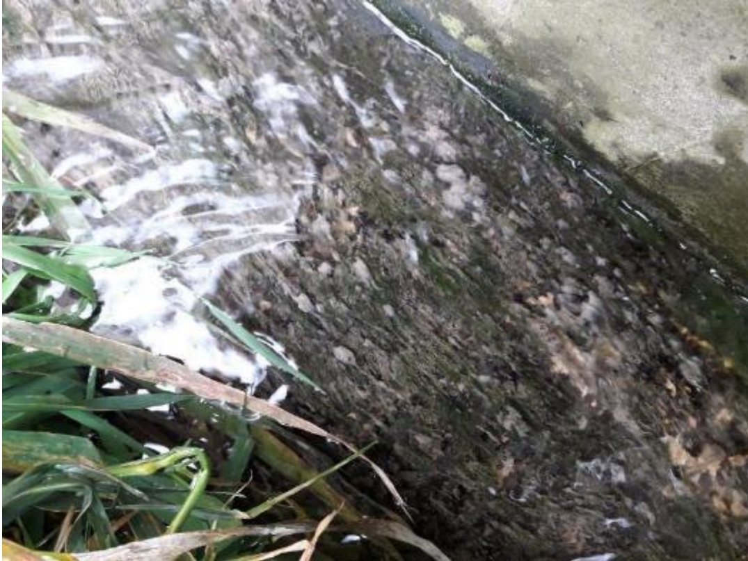
Figure 10: Unlicensed discharge flowing through a concrete culvert that enters the stream, just downstream of the location of Figure 9.
