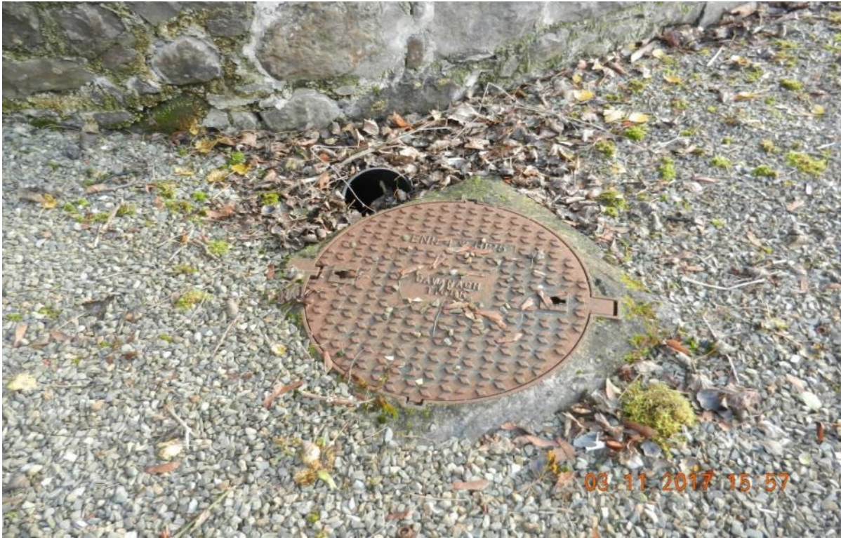
Figure 4-20: Bad Practice – Possible capacity issues – overflow from manhole is discharged to the receiving water (Photo: Joan Martin).
