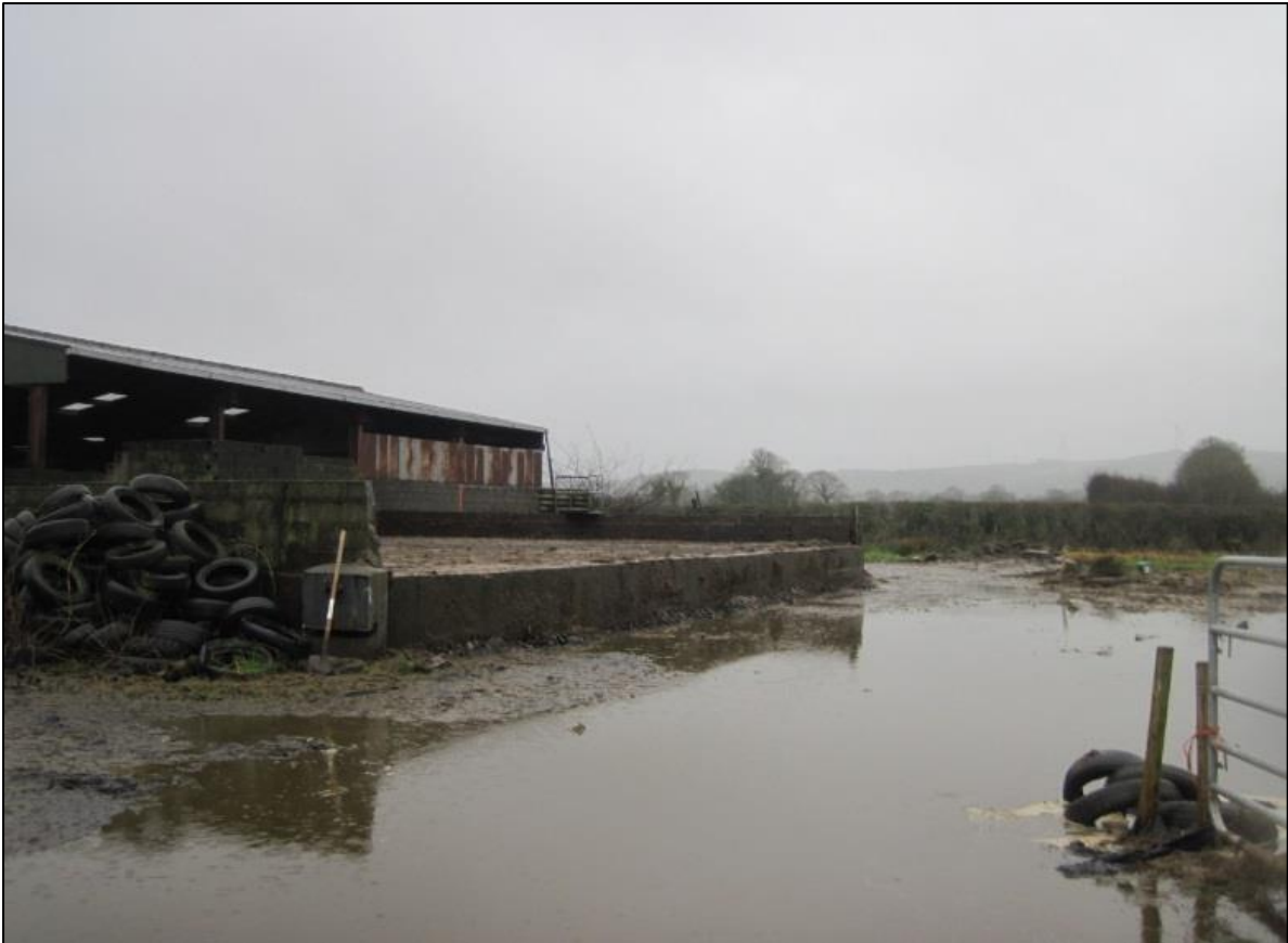
Figure 2-15: An extension to a slurry tank, approximately doubling its capacity, failed due to improper building techniques (Photo: Andrew Holmes).
