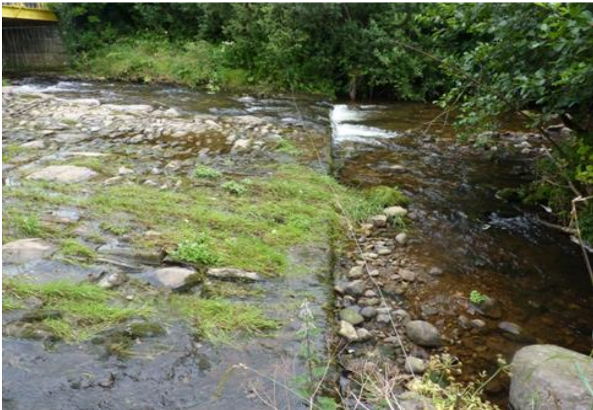
Figure 3-7: Example of the downstream section of a bridge apron. The height of the apron lip may impede the upstream migration of some fish species (Photo: Emma Quinlan).
