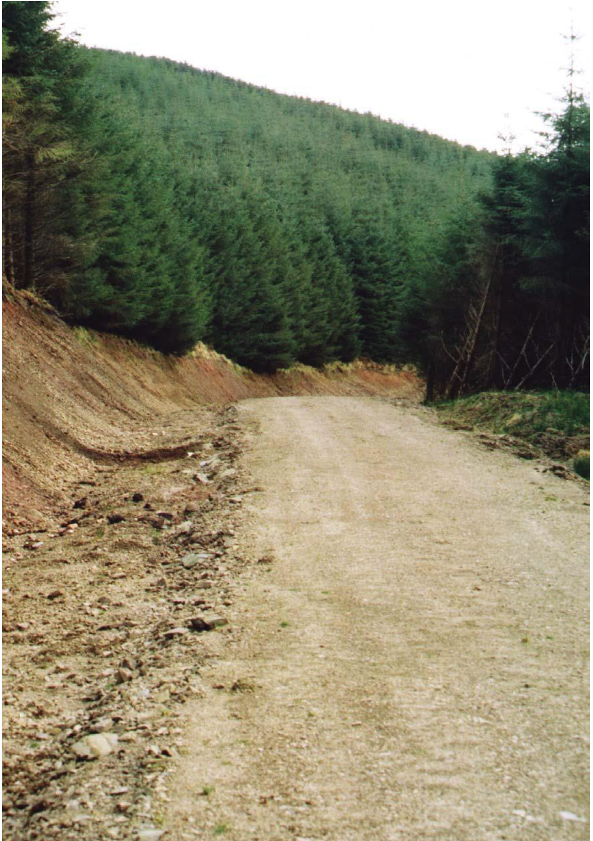
Figure 7-6: An appropriate forest road formation on a steep cross slope (Photo: Forest Service, DAFM).
