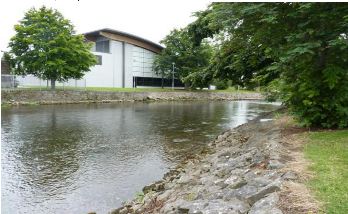
Figure 3-10: Examples of the use of rip rap as bank protection. By placing riprap along the river bank, this prevents lateral movement of the river and limits both riparian habitat and the input of sediment and wood (Photo: Emma Quinlan).
