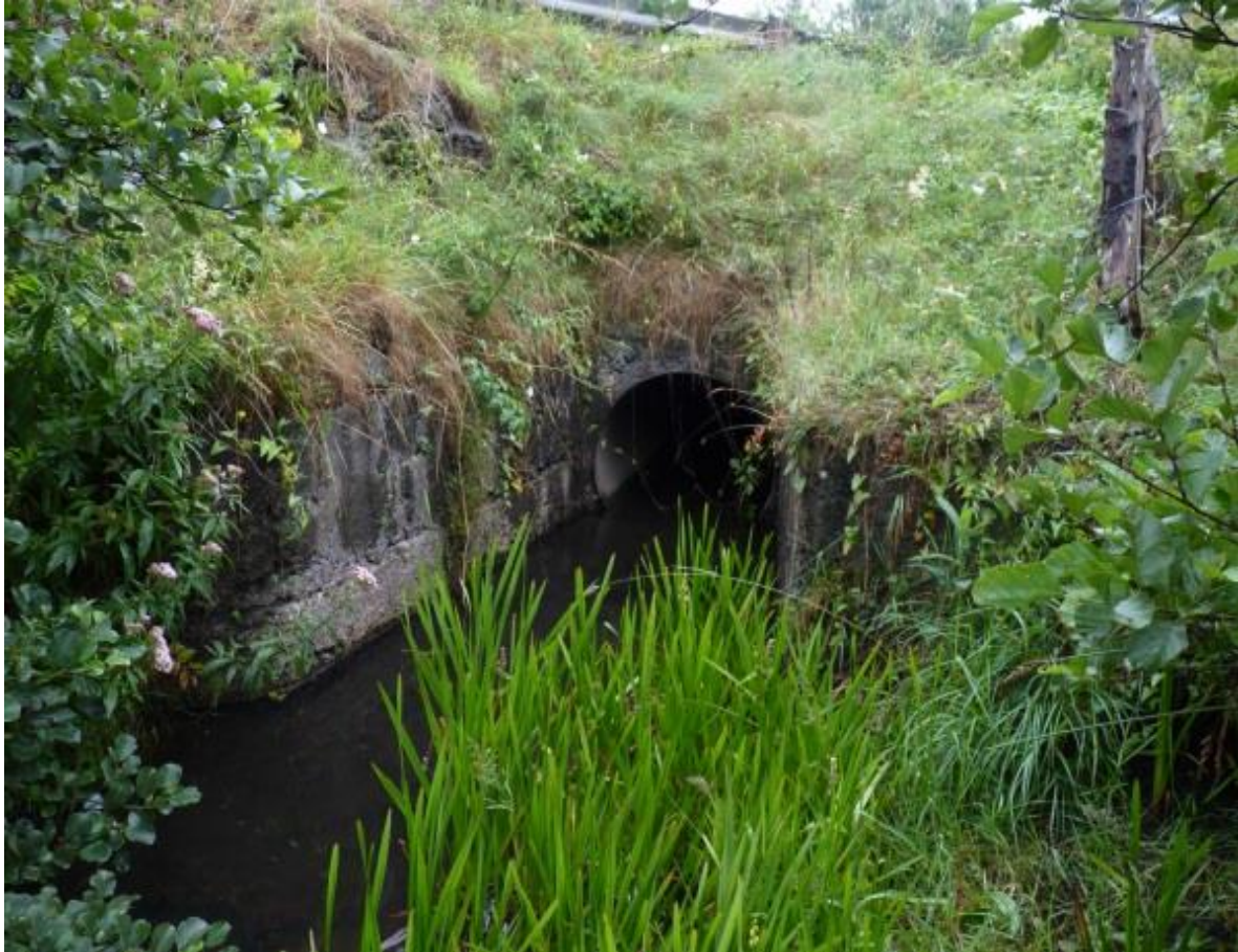
Figure 3-8: Example of a culvert. This structure will impede flow and the movement of sediment and fish (Photo: Emma Quinlan).
