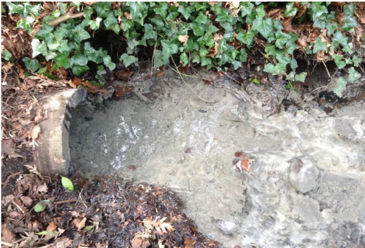
Figure 4-17: Discharge of raw sewage from a SWO during dry weather conditions – caused by a sewer blockage (Photo: Paul Buggy & Gerry O'Connell).
