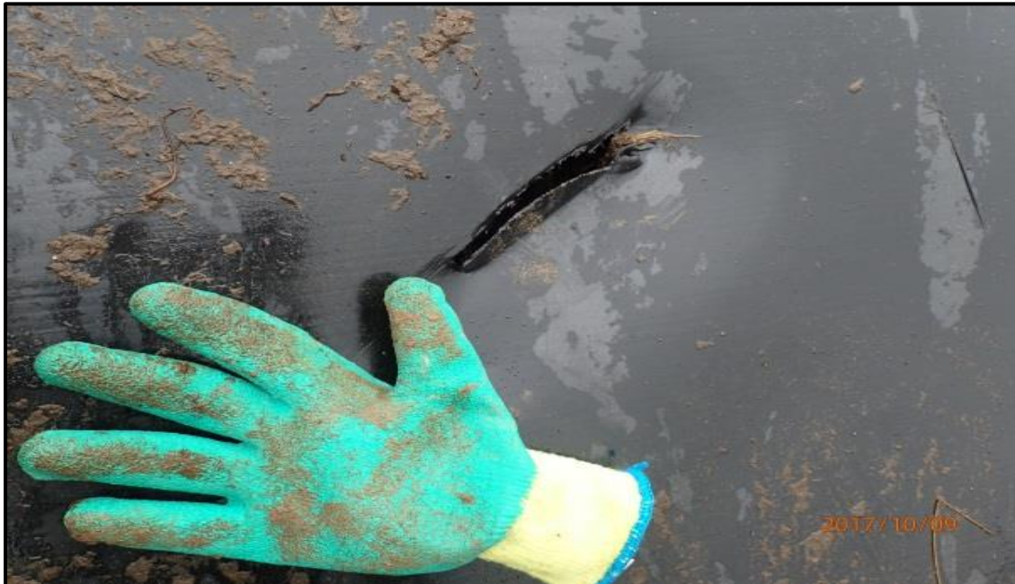
Figure 2-19: Tear in the geomembrane caused by a careless contractor when emptying the lagoon (Photo: Robert Imbusch).
