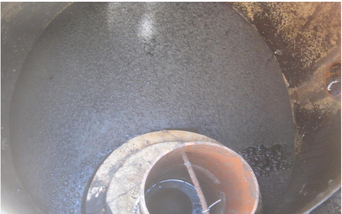
Figure 11-3: Interceptor on surface water drainage system. Note bubbles in the floating scum in the interceptor. Some scum on an interceptor surface is normal but presence of numerous bubbles such as this indicates an organic waste of some strength is entering the interceptor, with microbial degradation in the chamber resulting in gas bubbles. This would require further investigation into contamination of the surface water drains with an organic-type waste (Photo: Emmet Conboy).
