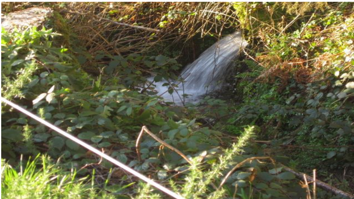
Figure 2-2: The presence of a very strong flow from a culvert indicates high hydrological connectivity (Photo: Mairead Shore).
