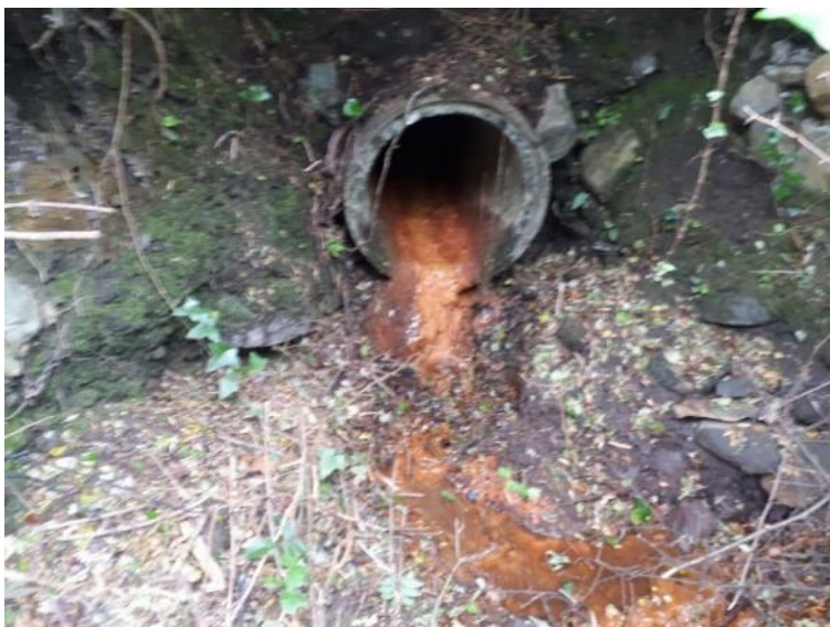
Figure 13.2: Leachate breakout from an unlined landfill (via an old stormwater pipe) (Photo: Kate Tynan).
