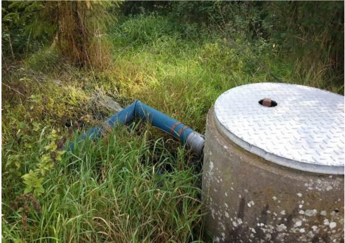
Figure 7-28: Unauthorised discharge point within a grant aided forest beside an IPC licensed facility (Photo: Thomas Sexton, EPA).
