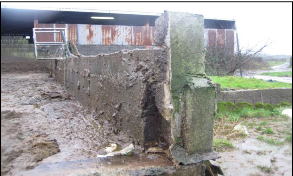
Figure 2-16: Close-up of the jointing area, where the extension wall was built on top of the existing tank with inadequate 'tie-in' between the new and old construction (Photo: Andrew Holmes).
