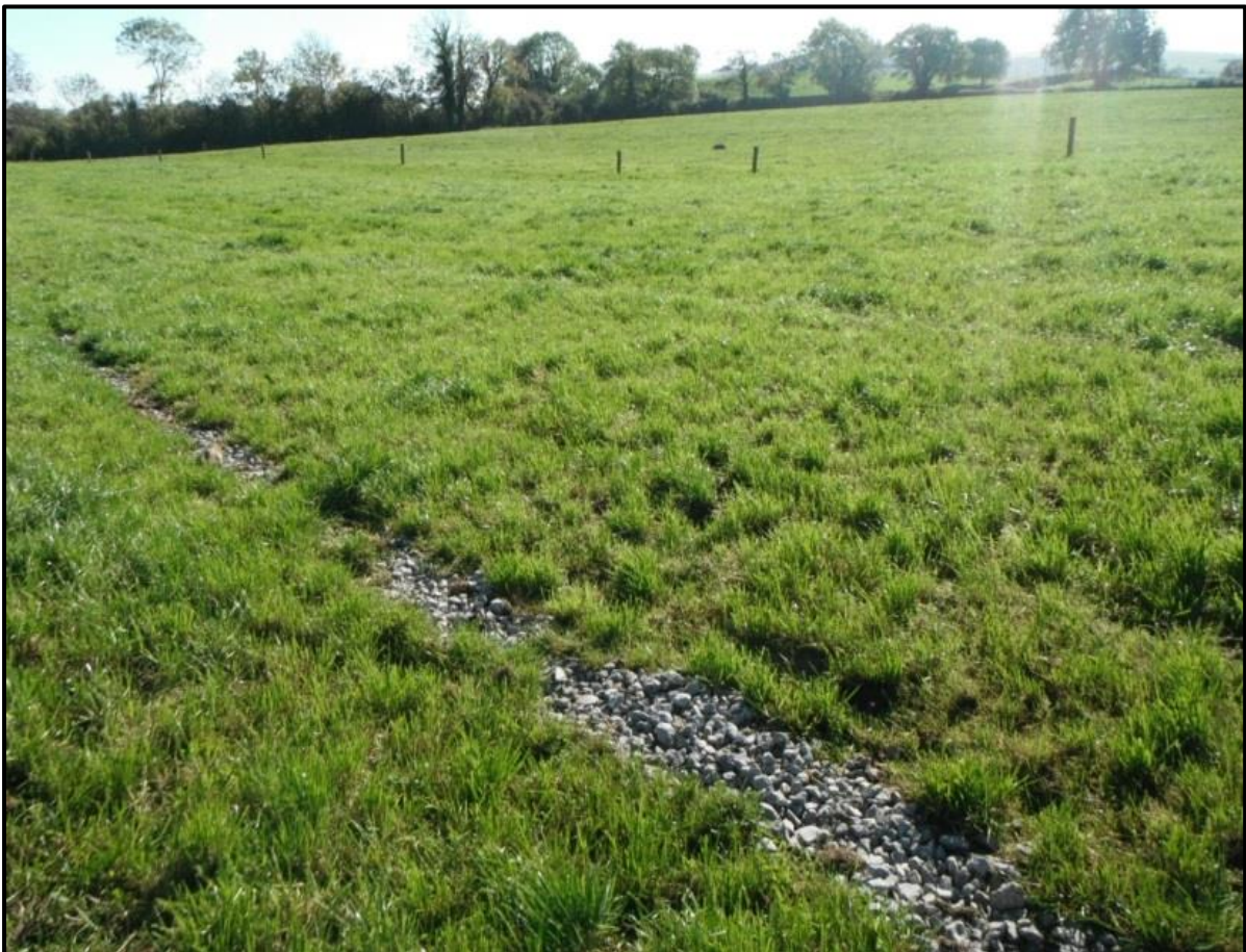
Figure 2-22: A pipe land drain which has been overfilled with stone providing a preferential pathway (Photo: Robert Imbusch).
