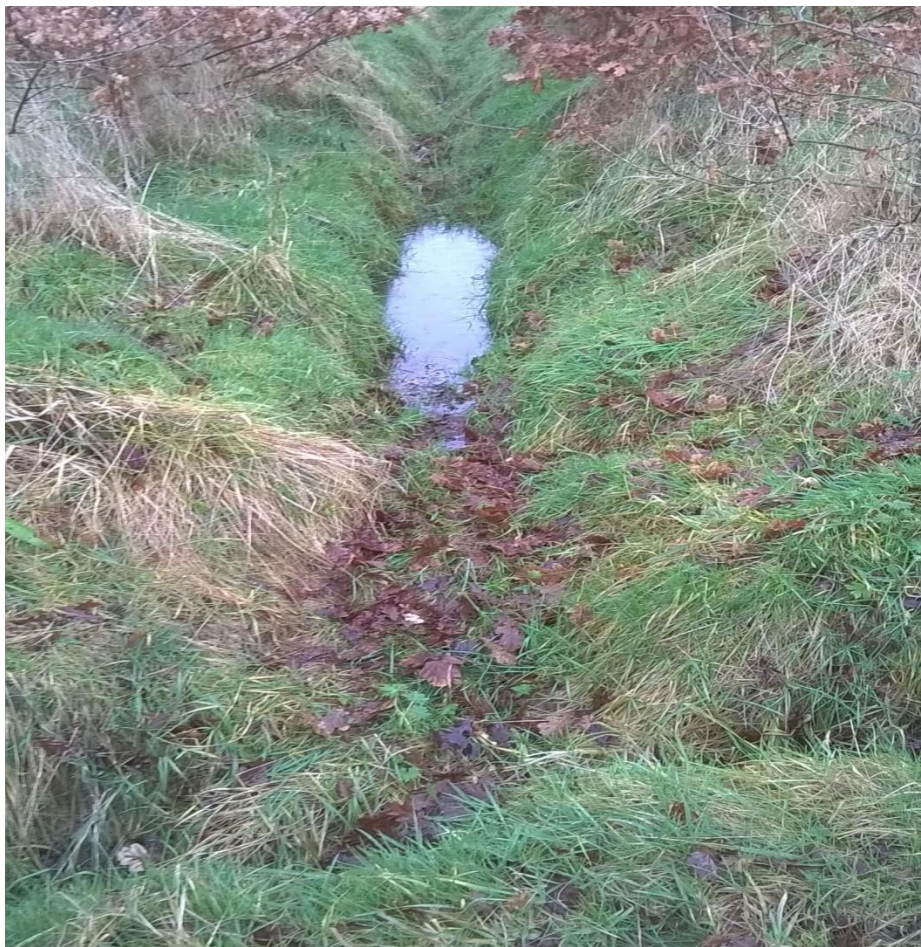
Figure 7-3: A functioning silt trap in a 'greened up' forest drain on a 4 year old afforestation site (Photo: Forest Service, DAFM).
