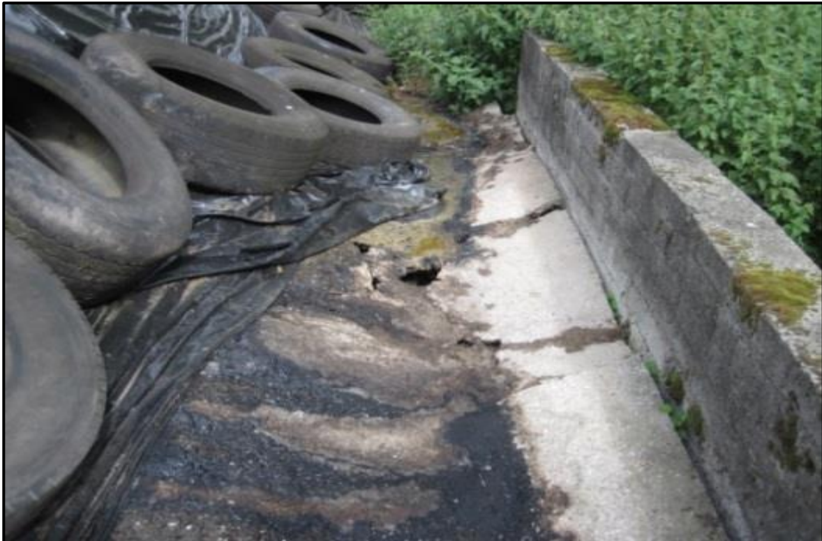
Figure 2-6: A cracked silage effluent channel allowing leakage (Photo: Andrew Holmes).
