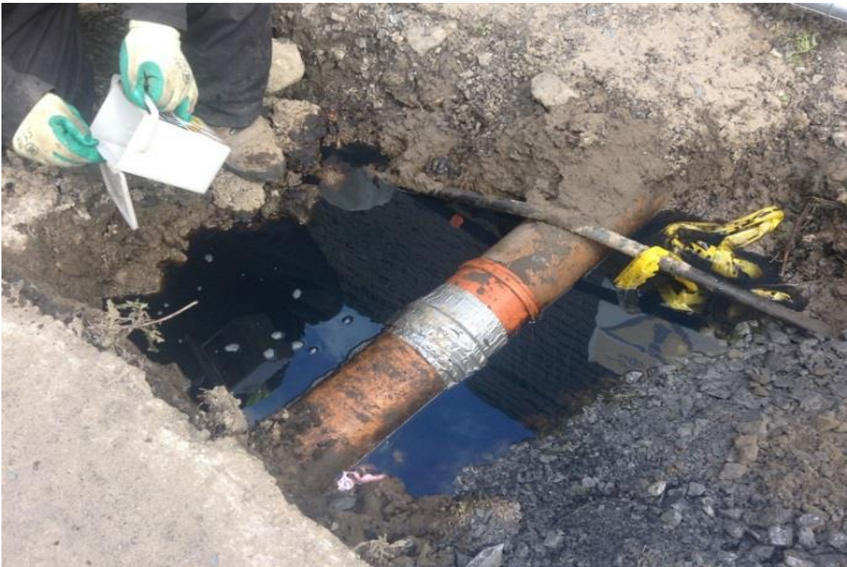
Figure 5-13: The oil entered the surface water system through a broken surface water pipe (now repaired) (Photo: Gerry Cullen).
