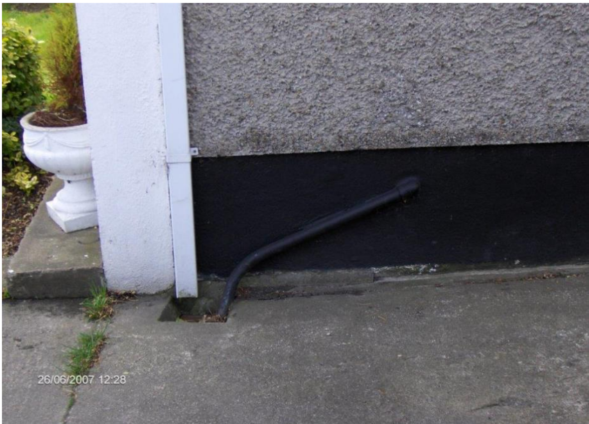
Figure 5-3: Misconnected drain to surface water gully (Photo: Tony Falkiner).
