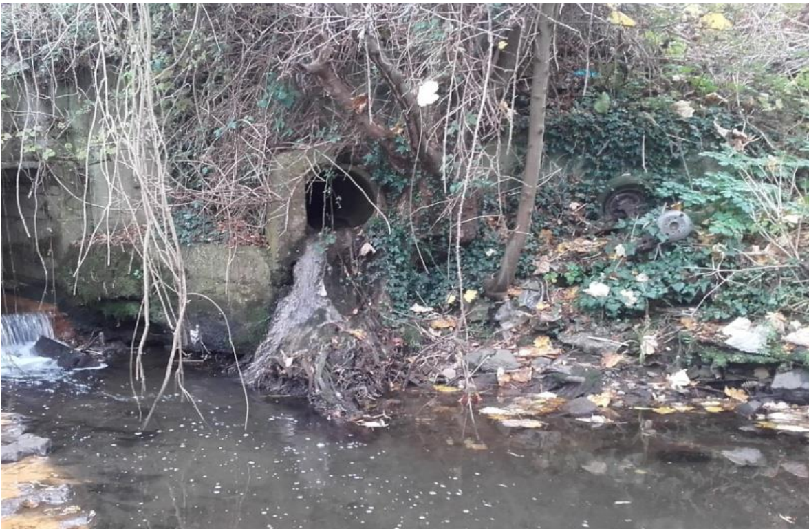
Figure 5-8: In this picture a surface water pipe discharges to the Dodder from approximately 1m above river level. Note the stream of sewage fungus that runs down the wall to the river – evidence of long term misconnections in the upstream catchment. (Photo: Paul Buggy).
