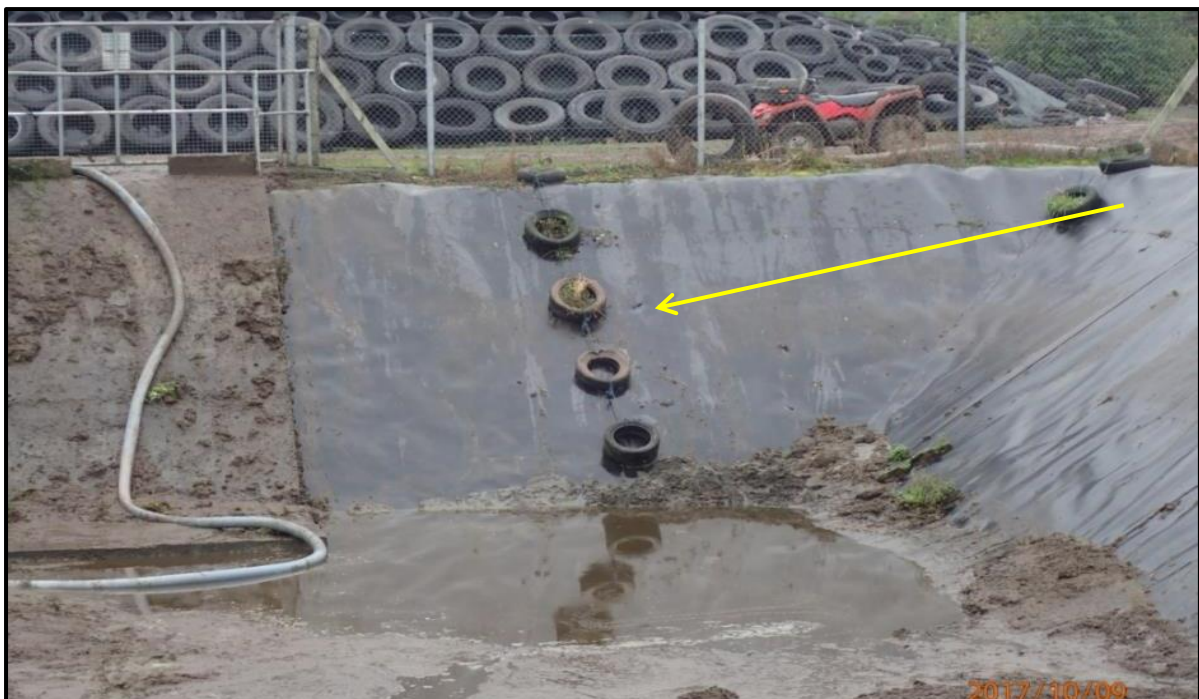
Figure 2-20: A tear in the geomembrane (shown by the arrow) caused 180 m 3 to discharge overnight into groundwater, and subsequently reappearing in a local stream 500 m away (Photo: Robert Imbusch).
