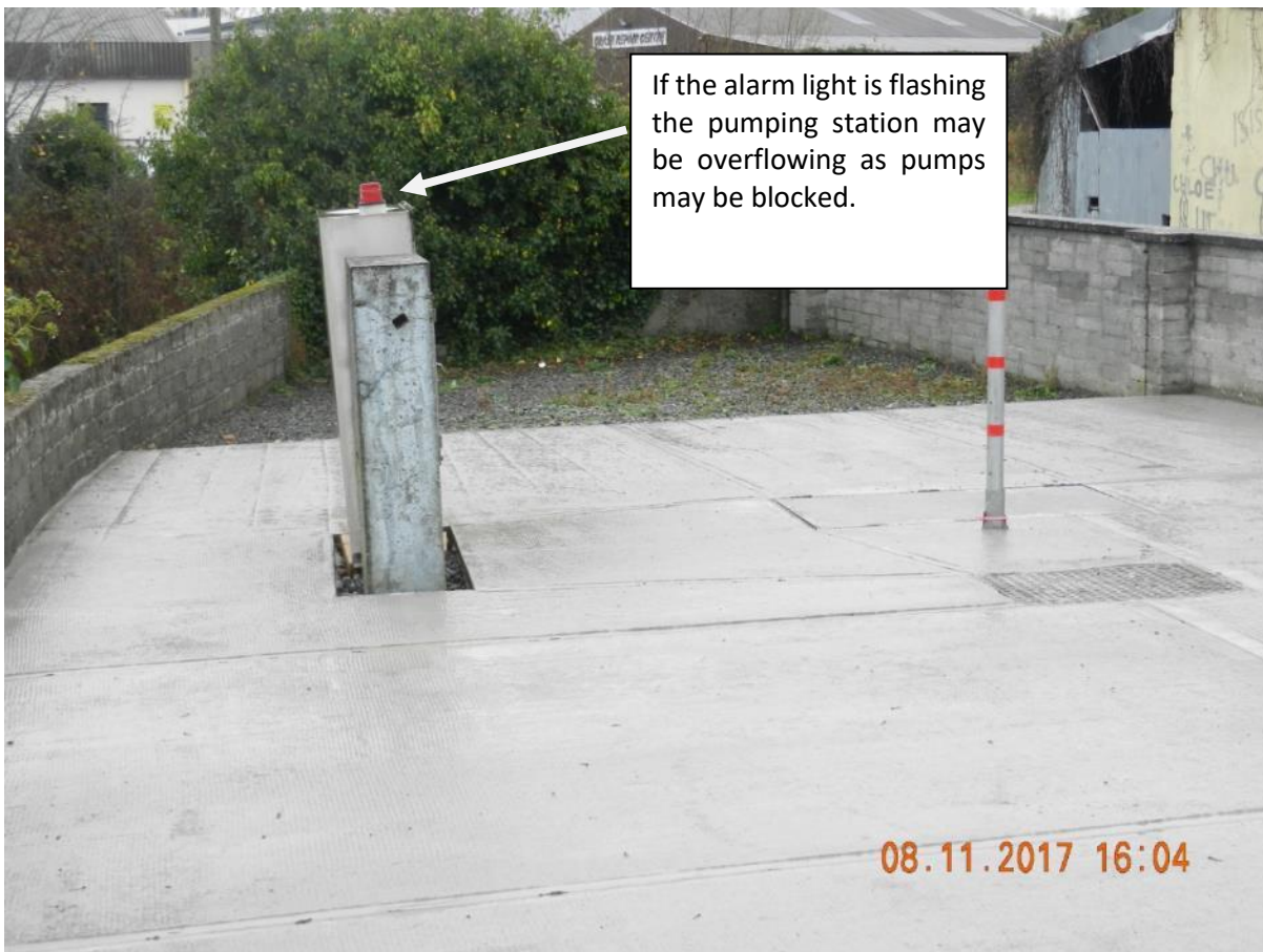
Figure 4-21: Good practice - Alarmed pumping station (Photo: Joan Martin).
