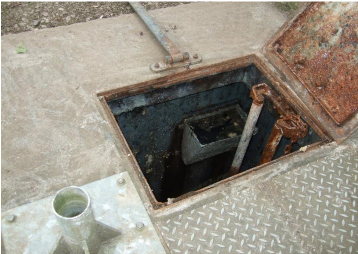
Figure 4-19: Typical pumping sump - Pumping stations usually has two pumps (duty and standby or duty/standby/assist in larger installations) which pump combined flows to the treatment plant (Photo: Joan Martin).
