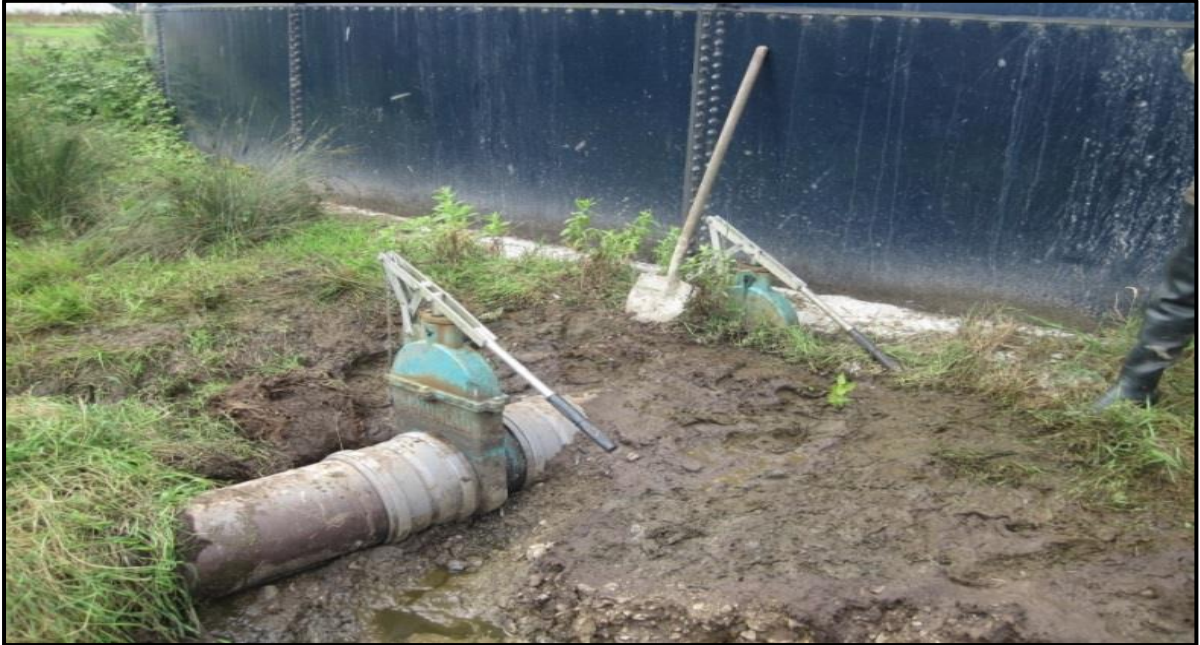
Figure 2-17: Failure to close the valve nearest the tank caused pressure to build up in front of the 2 nd valve. Because the second valve wasn't set in concrete, the valve was pushed out and slurry discharged from the breach in the pipe just before the 2 nd valve (Photo: Andrew Holmes).
