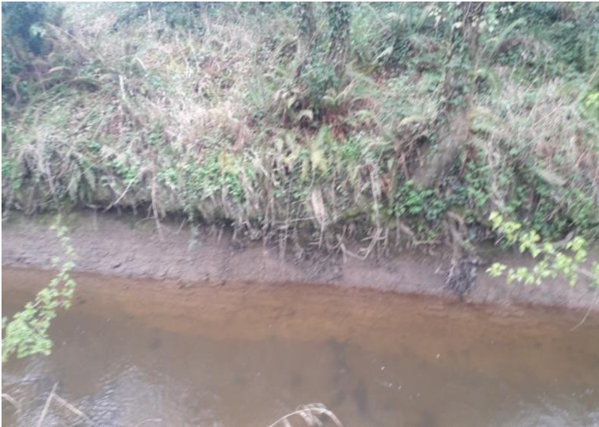
Figure 2-4: Bank undercutting – may cause bank collapse (Photo: Mairead Shore).
