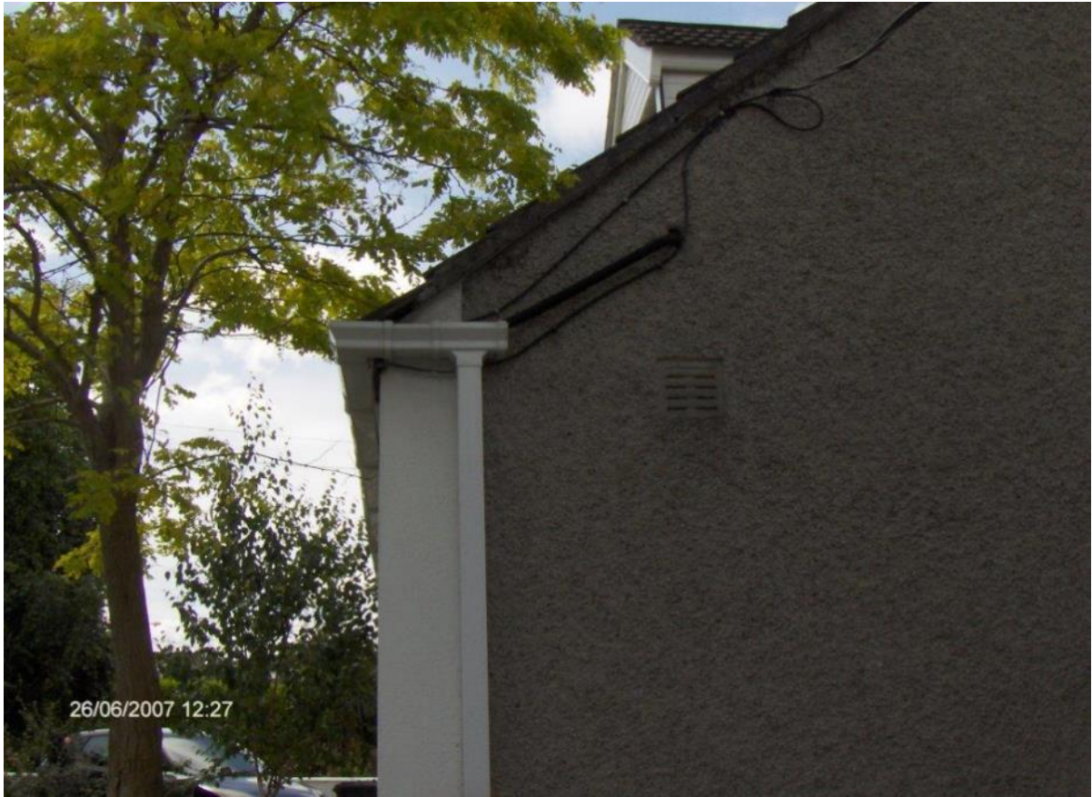
Figure 5-4: Misconnected pipe to gutter (Photo: Tony Falkiner).
