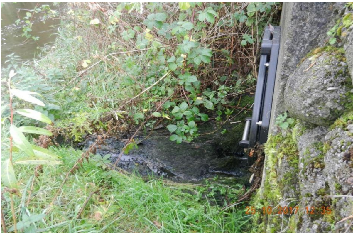
Figure 4-8: Good Practice - Storm water discharge point. Note that it is not discharging in dry weather and there is no indication of solids in the immediate discharge vicinity which indicates good practice and indicates that the storm water has been screened and settled in a tank prior to discharge (Photo: Joan Martin).
