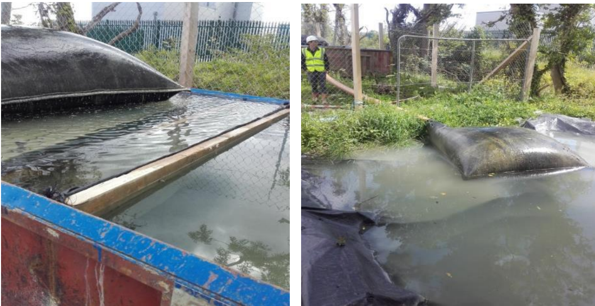
Figure 5-16: Dewatering for basement construction. Silt contaminated groundwater is treated by means of 2 settling tanks (with baffles) in series, each with filter bags at the entry to the tanks. Final effluent is discharged to the local stream. Discharge is subject to a Section 4 effluent licence (Photo: Gerry Cullen).
