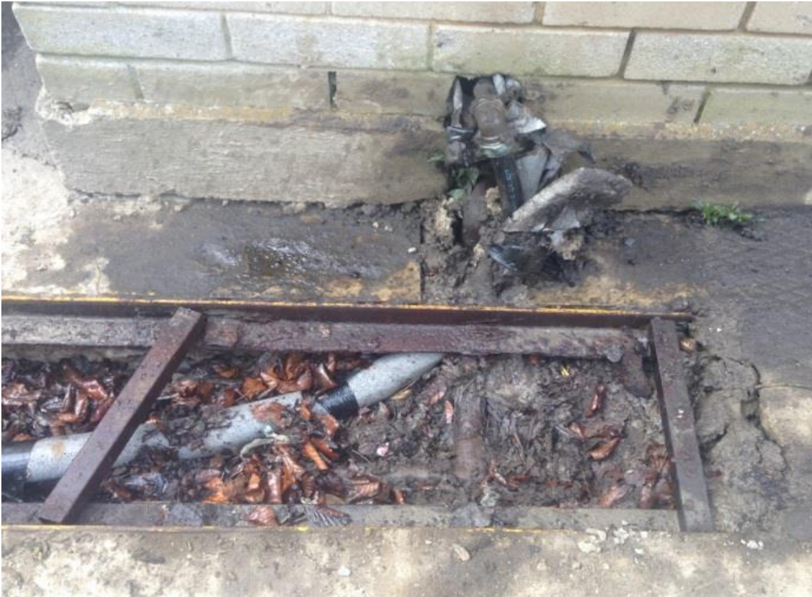
Figure 5-12: Leaking oil pipe between the tank and boiler at a swimming pool. (Photo: Gerry Cullen).
