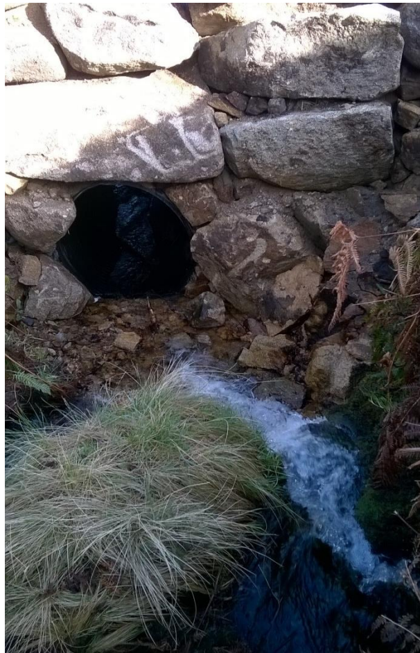
Figure 7-8: A culvert pipe installed under a forest road to facilitate passage of a stream (Image: Forest Service, DAFM)
