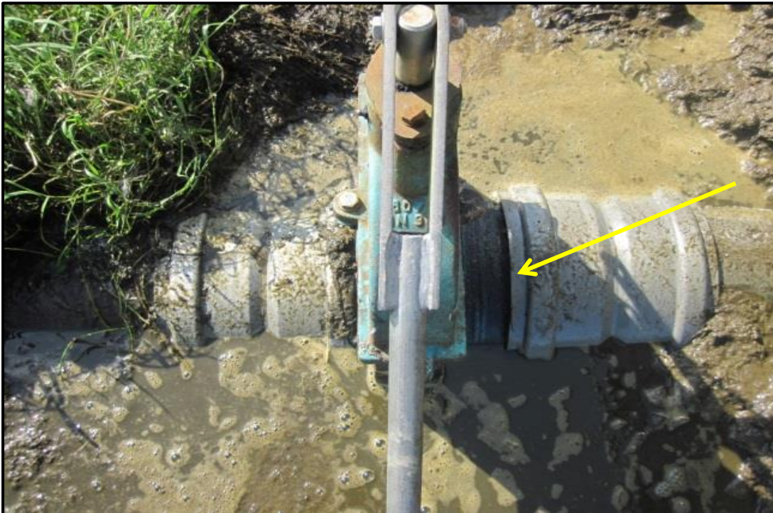
Figure 2-18: The arrow point to the area where the valve was pushed off the pipe and the leak occurred (Photo: Andrew Holmes).
