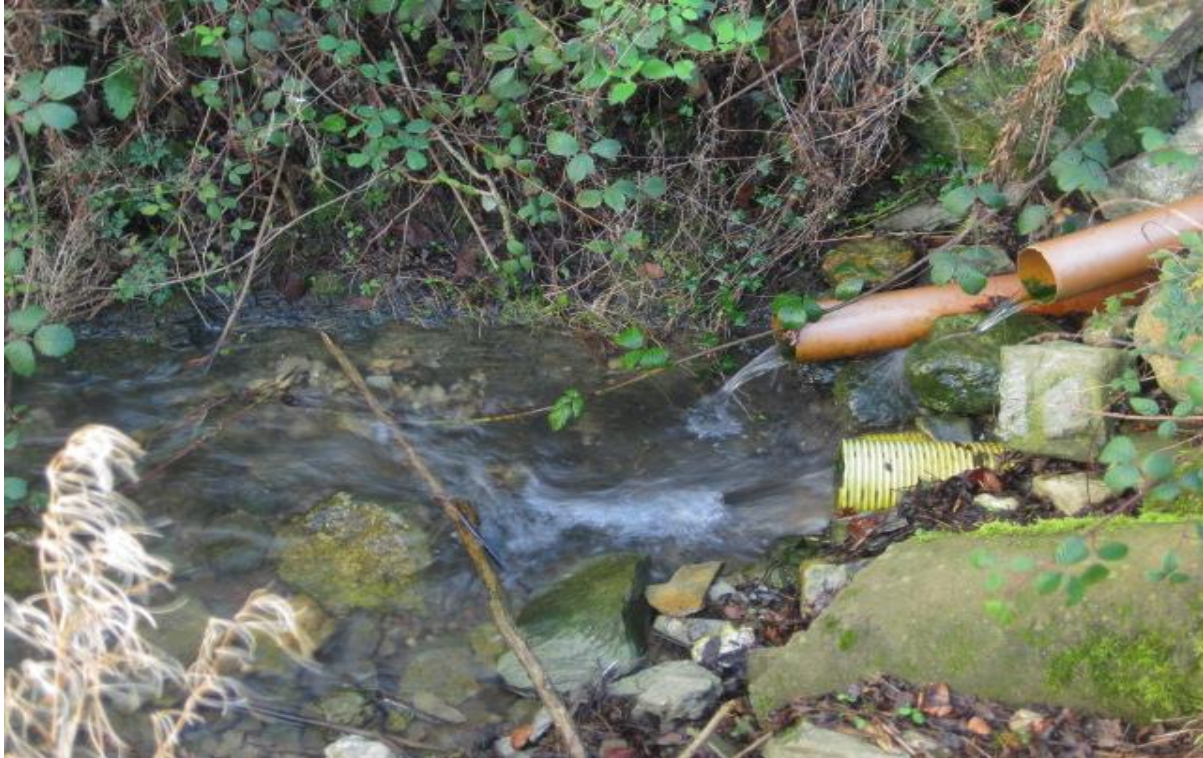
Figure 2-1: The presence of 3 flowing culverts here indicates high hydrological connectivity (Photo: Mairead Shore).
