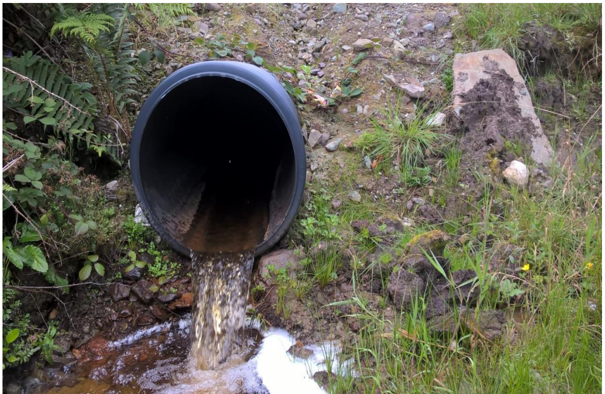
Figure 7-10: Forest road culvert to facilitate the crossing of a small stream, with an inappropriate step preventing fish movement upstream (Photo: Forest Service, DAFM).
