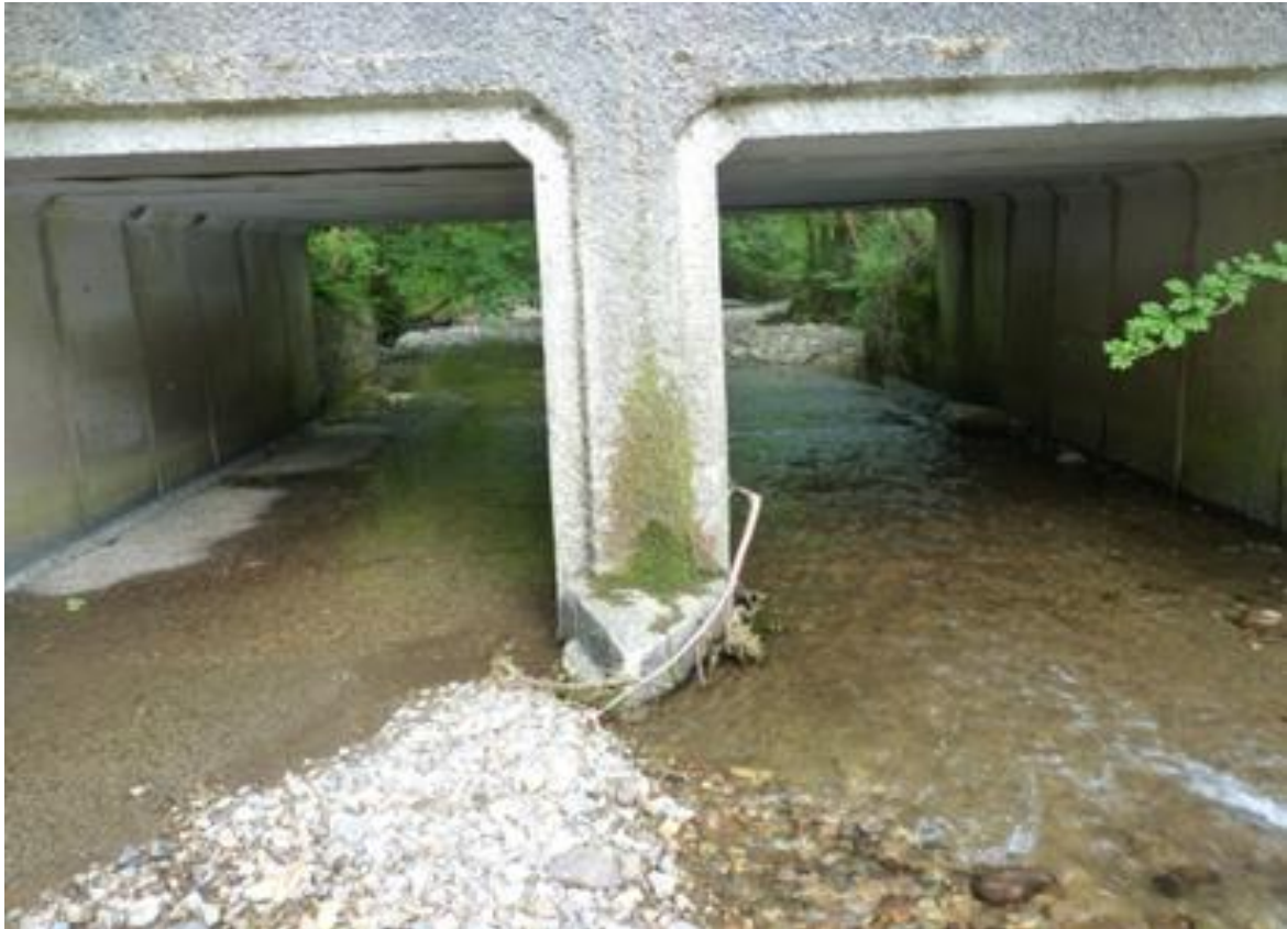
Figure 3-6: Example of a bridge apron. This will impede the movement of sediment and fish passage (Photo: Emma Quinlan).
