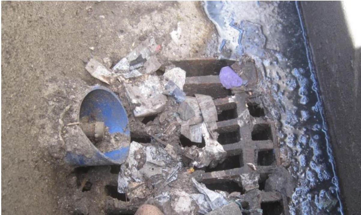
Figure 11-4: Outlet drain fitted into base of bund around above-ground wastewater storage tank. Note outlet leads to surface water gully. The outlet connection creates a high risk to waters as it could potentially be used to facilitate emptying polluted contents from the bund into storm drains. Outlet should be removed / sealed (Photo: Emmet Conboy).
