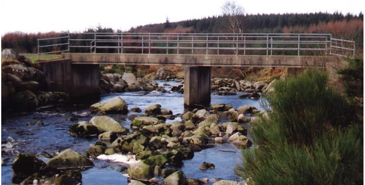
Figure 7-7: A concrete beam forest bridge with adequate clearance for storm events (Photo: Forest Service, DAFM).
