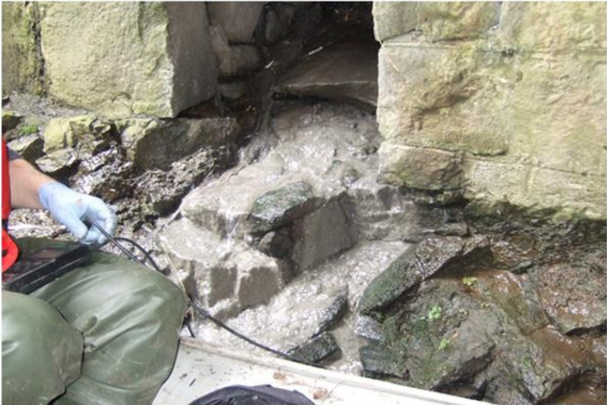
Figure 4-16: Storm water discharge on a combined network. Note physical discolouration of rock with indicates repeated contaminated overflows. CCTV surveying will be required in this instance to locate the SWO (Photo: Joan Martin).
