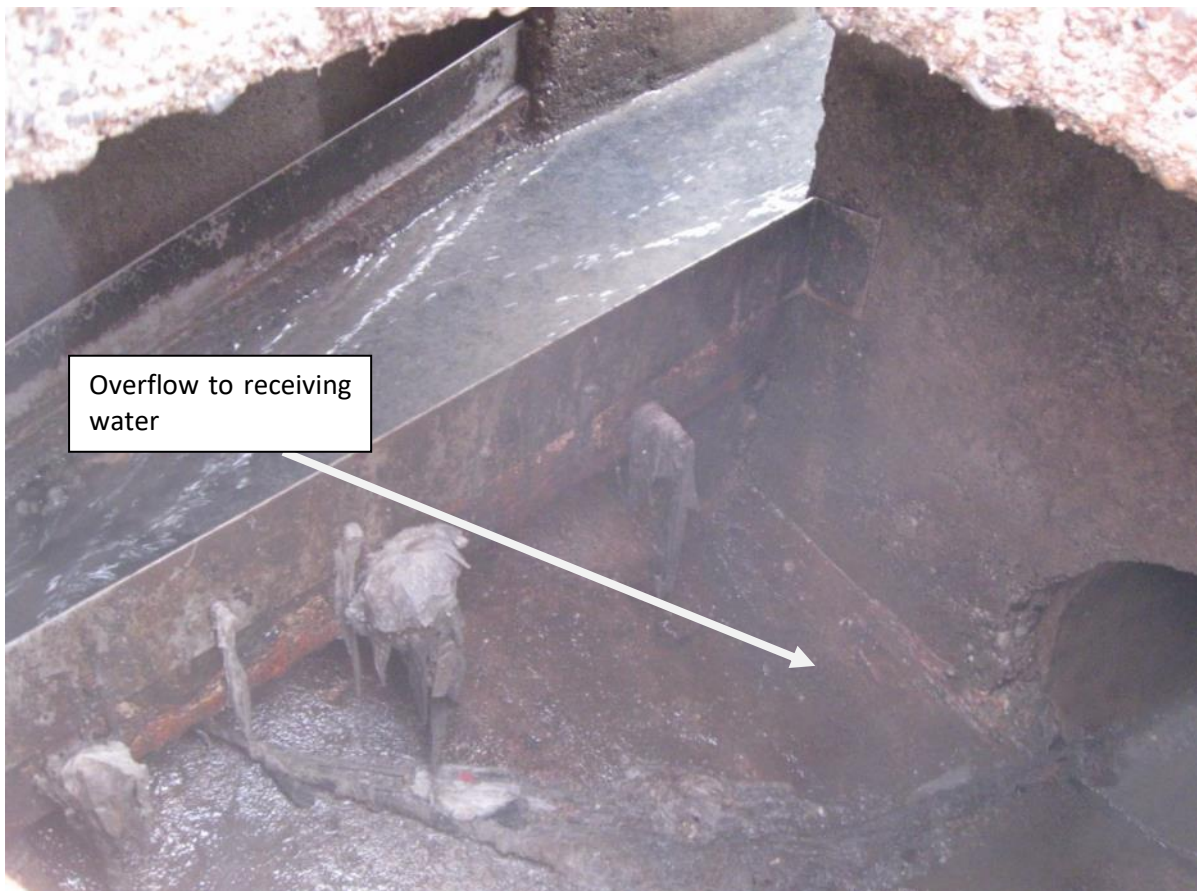
Figure 4-11: Bad Practice – Example of a SWO on a combined network. Note the overflow pathway to the receiving water which receives no screening (Photo: Joan Martin).
